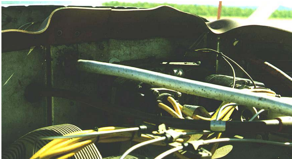
Figure 6-26. Improperly Positioned Aft and Side Peripheral Baffle Seals
