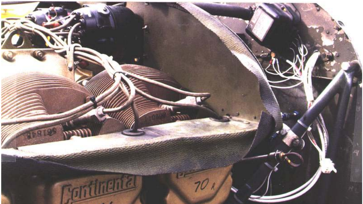
Figure 6-24. Improperly Positioned Baffle Seals
