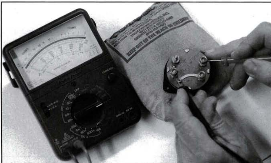
This photo shows the left mag circuit being tested with the mag in the "Left" mag position. The ohmmeter shows no needle movement, indicating the circuit is "open" and working properly.
