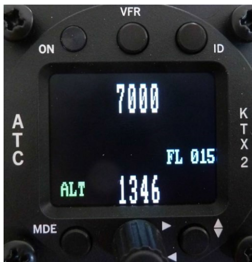
No GND switch installed
