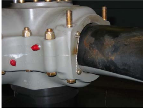
FIGURE 2-1. Grease Leak Residues
